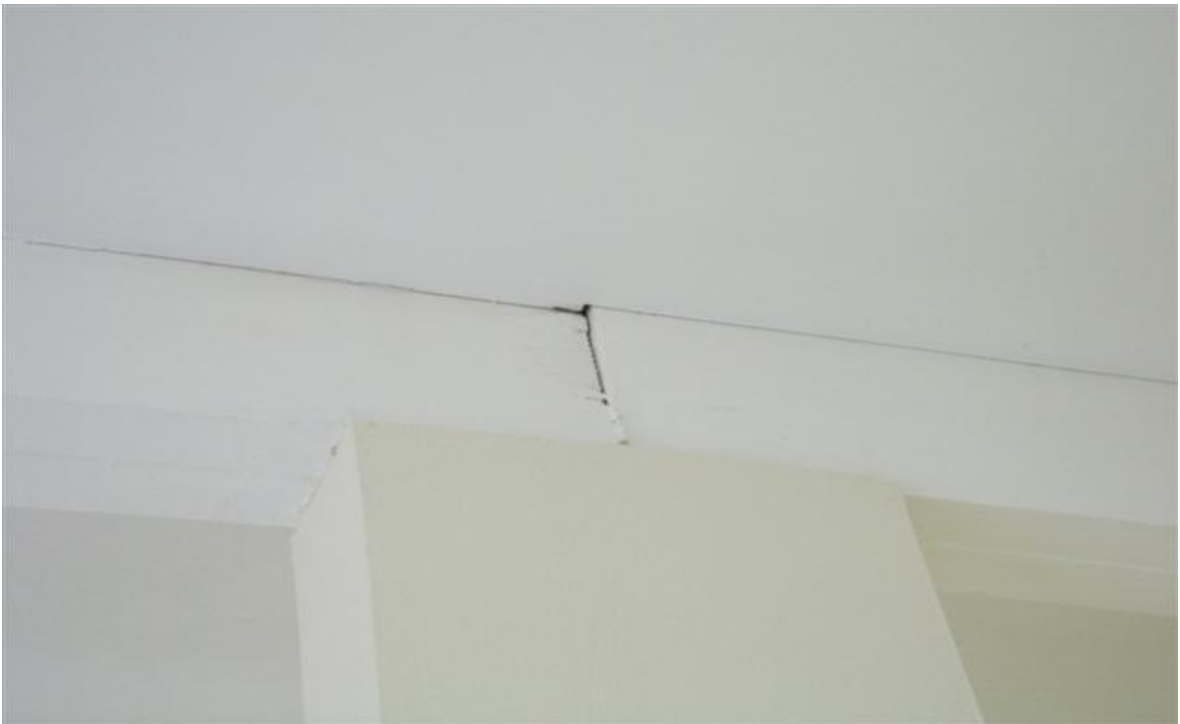
Figure 7c. Picture showing some damage on the inside structure of the house.
