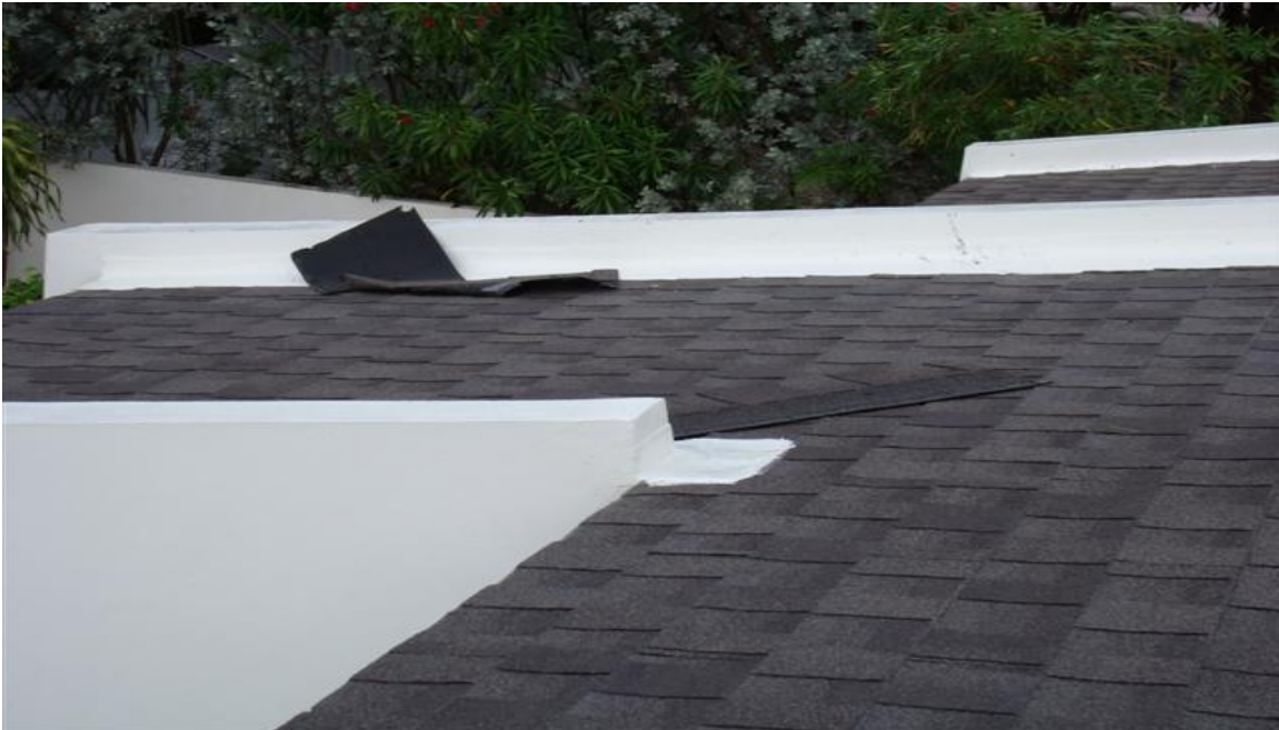
Figure 7a. Picture showing some roof shingles blown away.
