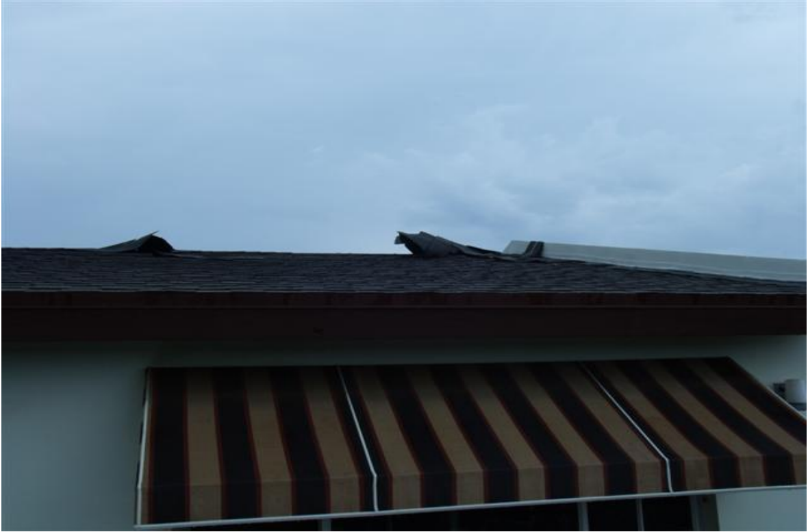
Figure 7b. Minor damage caused to the roof.
